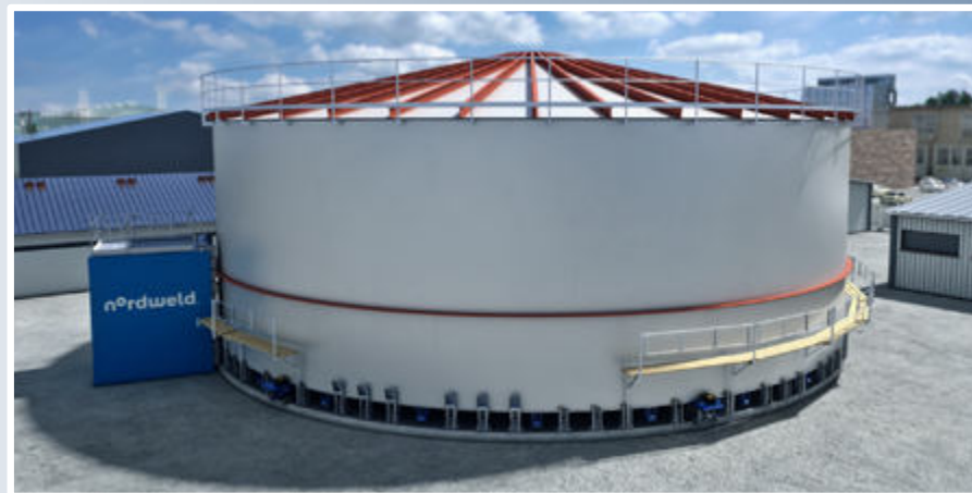
8. Assemble the 3rd course and so on until the tank reaches the final height.
